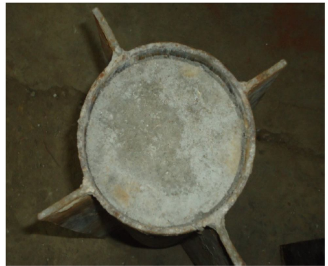
Fig 5. Typical bond failure of CFT
