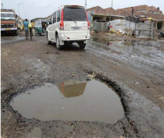
Photo 1 Water logging problems with Flexible Pavements
