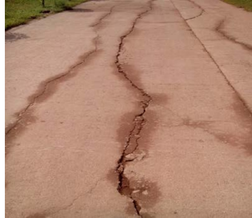
Photo 2 Cracks in Rigid Pavement
