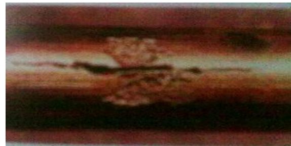
1.1a. A typical case of Failed Tube as a result of Stress Corrosion Cracking
