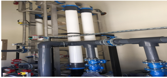
Fig.8 MBR pilot plant test white columns represent membrane skid
