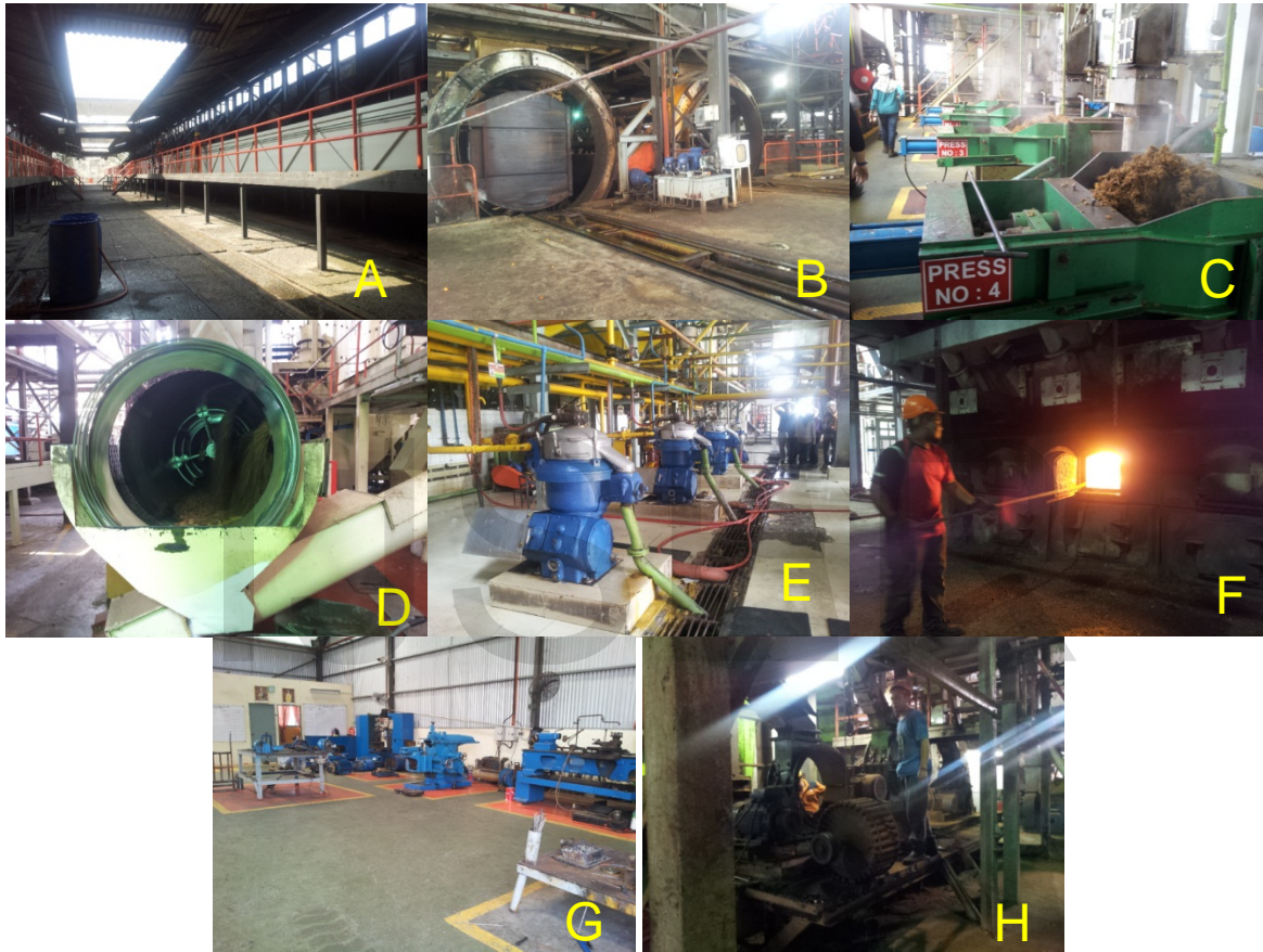
Figure 1: A) Loading Ramp, B) Sterilizing, C) Pressing, D) Nut Plant, E) Clarification, F) Boiler Room, G,H) Workshop
